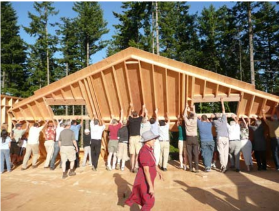
Chamber members join together to raise a wall of the new education center at Hopkins Demonstration Forest.
